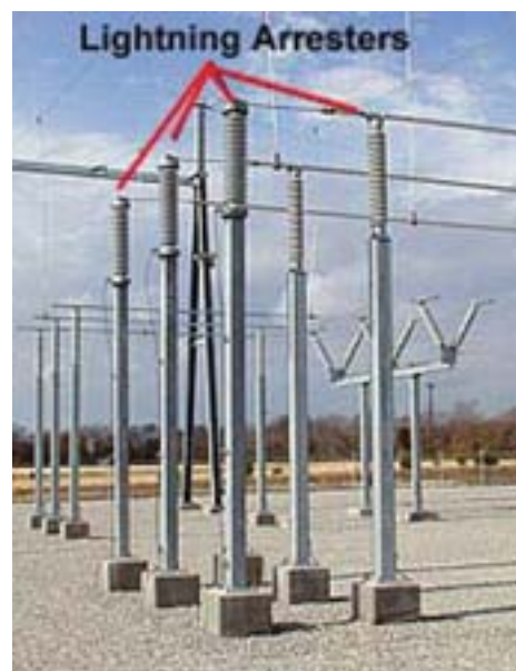
Lightning arresters on bus structures
